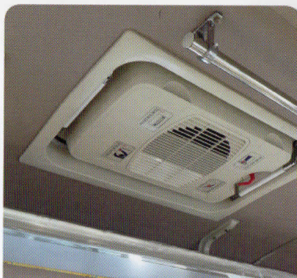
Emergency Exit With Roof Ventilator
